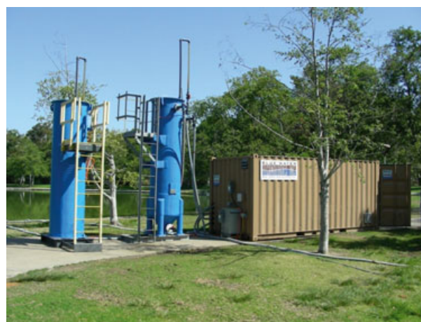
Fig. 1. Temporary Blue Pro™ water treatment facility at Mason Lake, April 2008. In a permanent facility, the sand towers can be embedded in the ground, and the trailer can either be camouflaged or decorated as an attraction for public education.
